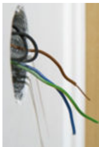
Exposed electrical wires.
